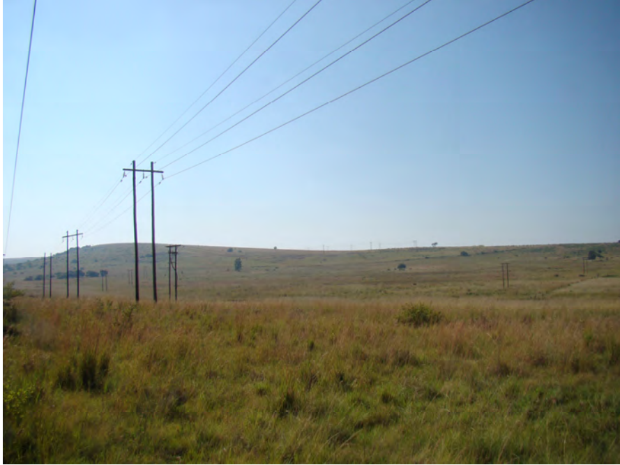
Fig. 3: B-C-D: This area has existing power lines and is situated in wetland.
