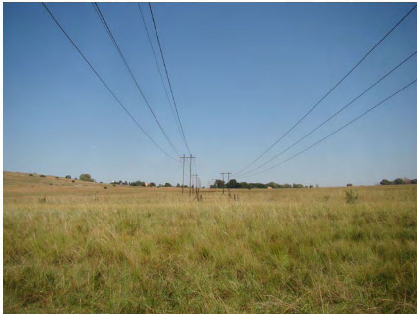
Fig. 2: A-B: Doornpoort substation is at the top of this hill. This area has existing power lines. The area is situated in wetland.
