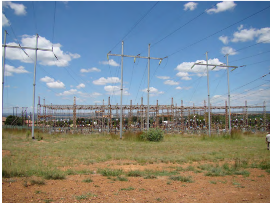
Fig. 27: Middelburg substation. The proposed new line will go in a westerly direction for 1 km to a new substation.
