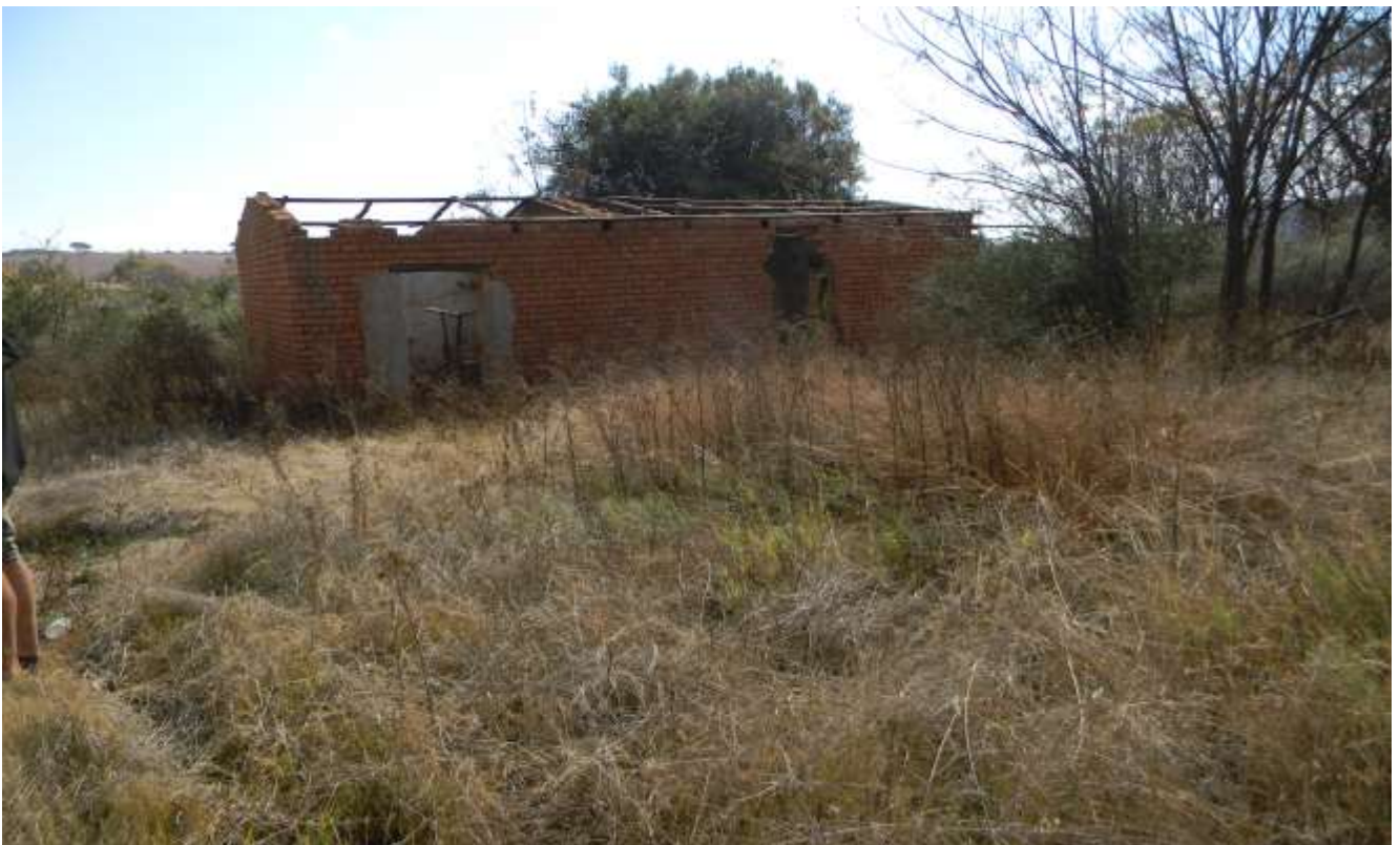
Plate 41: Photo 41: Showing a dilapidated farm building (Photograph © by Author 2021).
