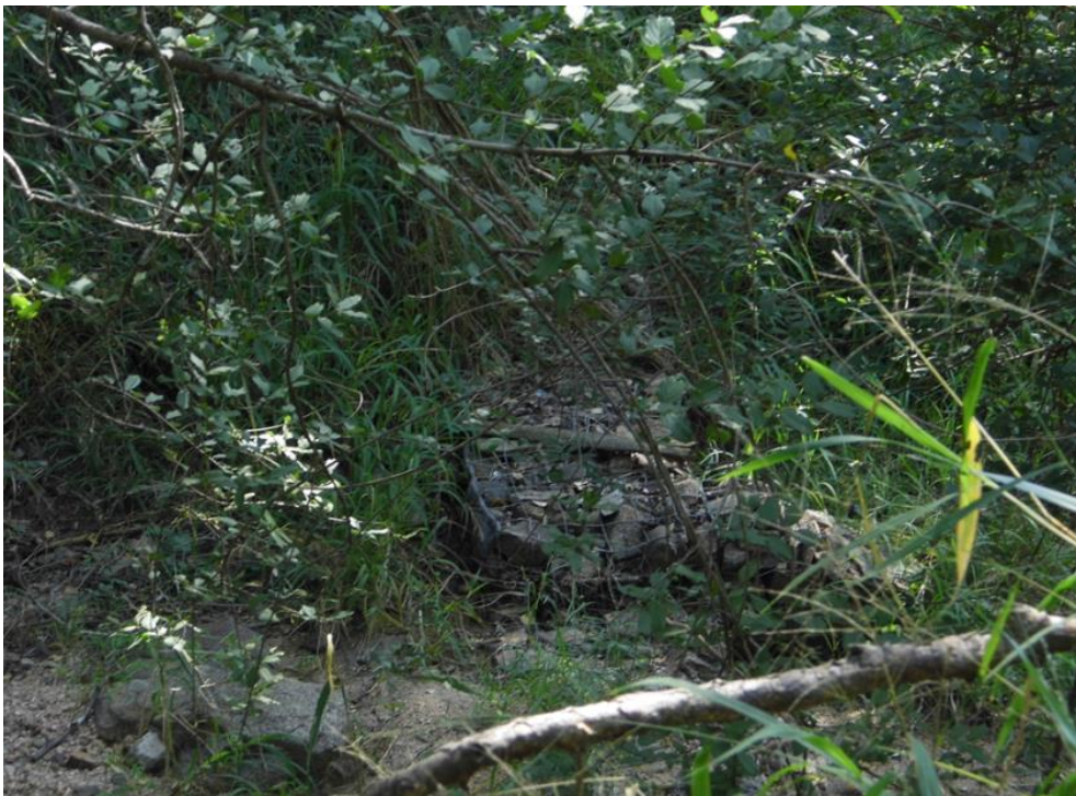
FIGURE 27 EXISTING GABBIONS THAT COVER THE EXISTING CABLING.
