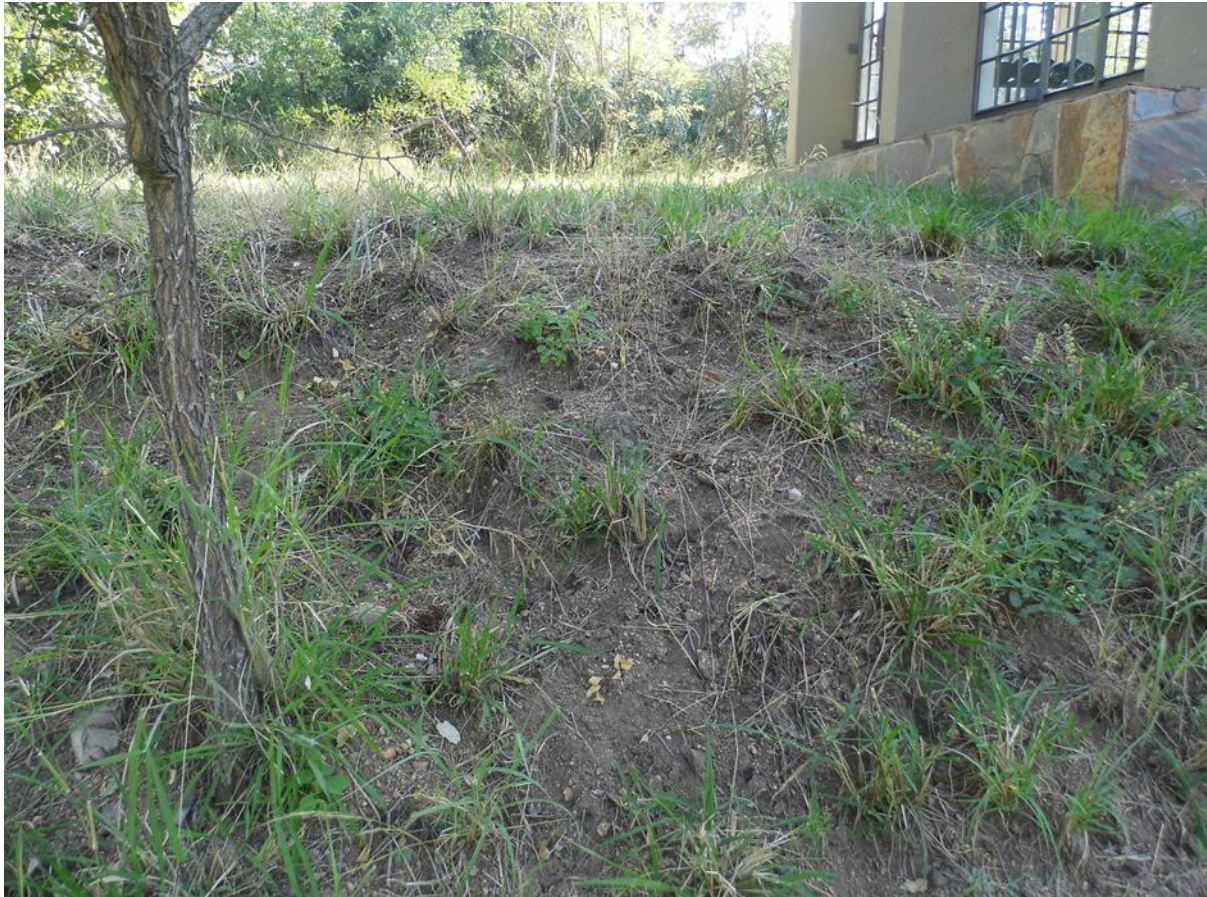
FIGURE 40 THE VERTICLE EMBANKMENT CUT INTO THE GROUND DURING THE CONSTRUCTION OF THE TENNIS COURT.
