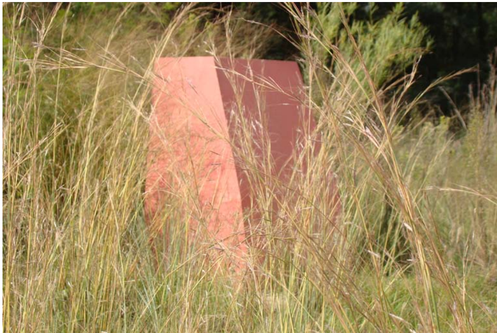
Fig. 4: Concrete markers to identify the SASOL gas line.
