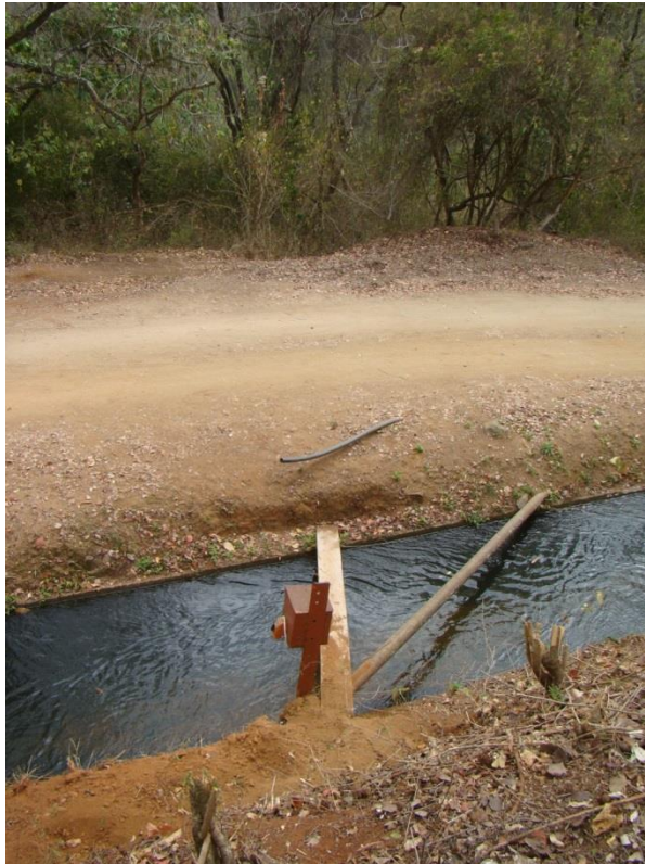
Fig. 22: The new line will cross the existing road and canal at this point and follow the route to the hydro building.
