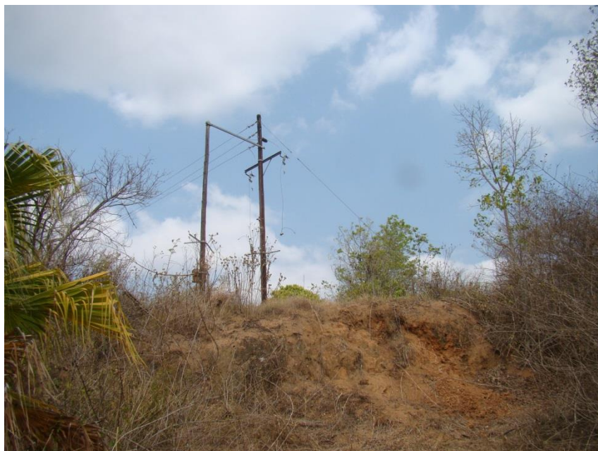
Fig. 19: The end of the existing powerline close to the ruin of the farmhouse.
