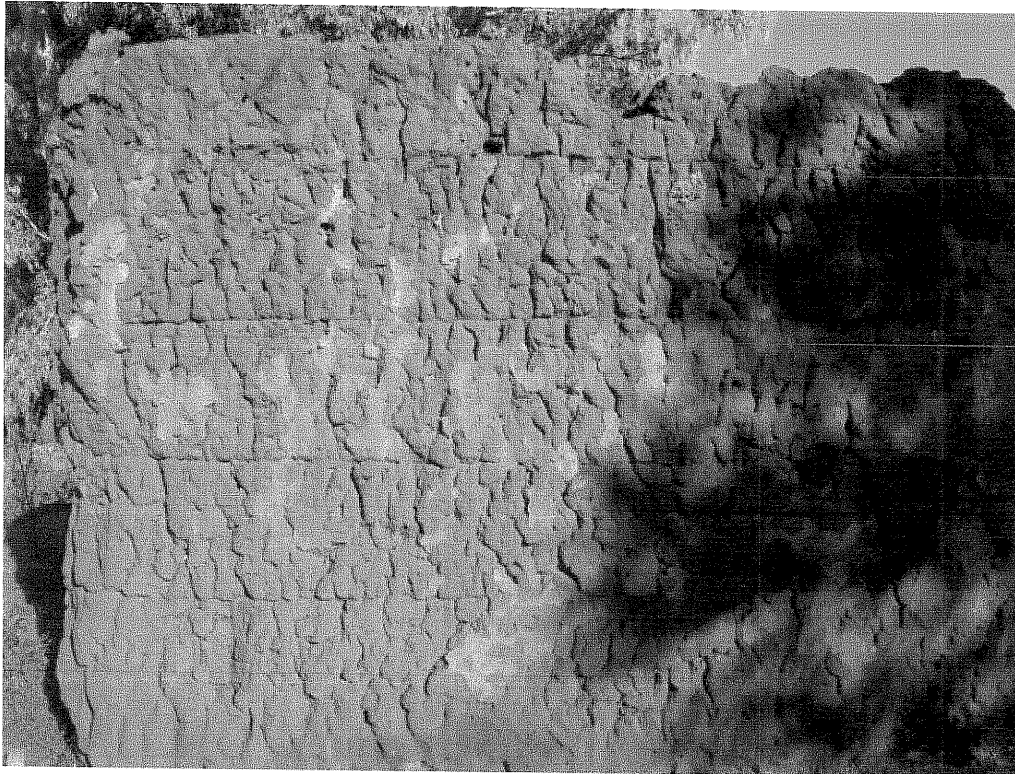
No. 7 Close-up photograph of one of the clay walls. The different layers of clay are still visible.
