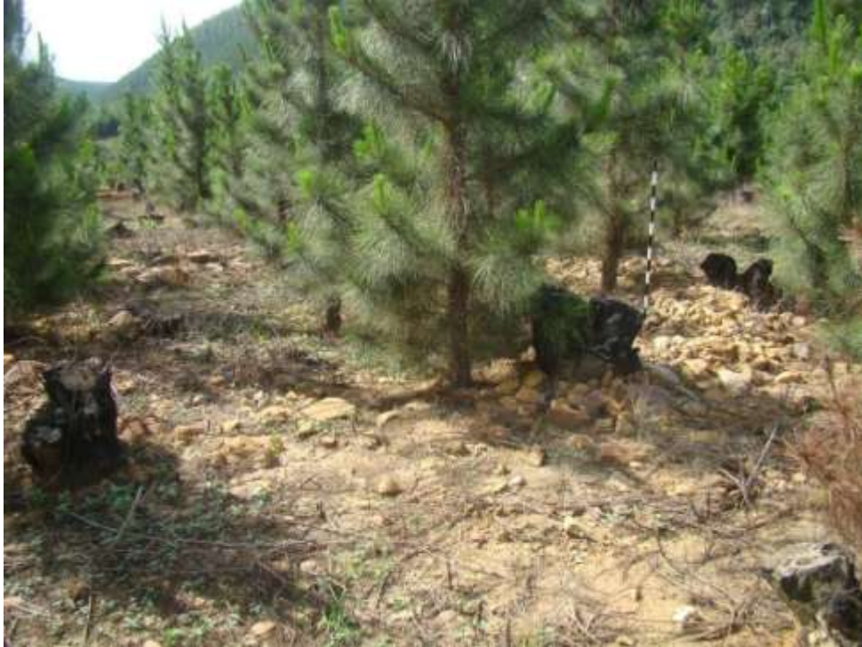
Fig. 34: The walls have been damaged severely by the plantation in this section.
