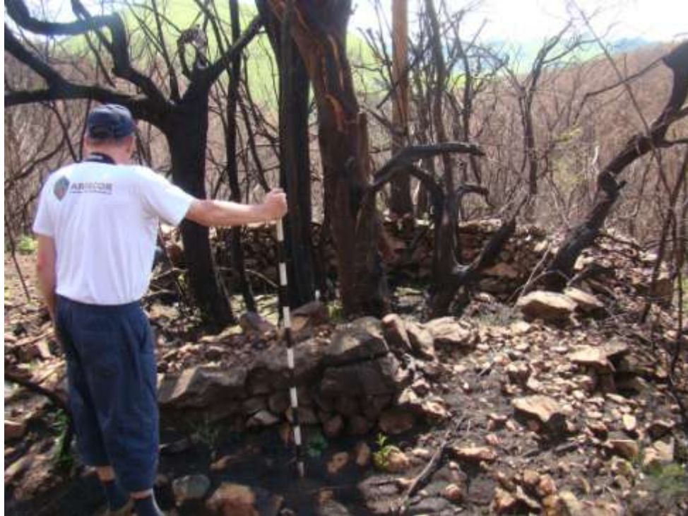
Fig. 198: One unit on the edge of the valley is in a fairly good condition, but natural vegetation is growing inside the wall.
