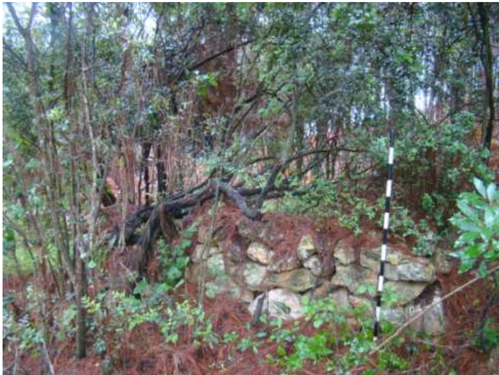
Fig. 58: A circular stone wall which is still in good condition. Sections of this wall are approximately 800mm high. The wall is covered with pine needles and overgrown with vegetation.
