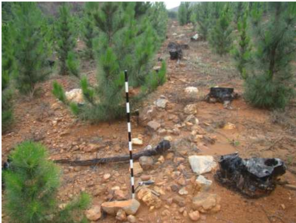
Fig. 49: A deteriorated terrace wall.
