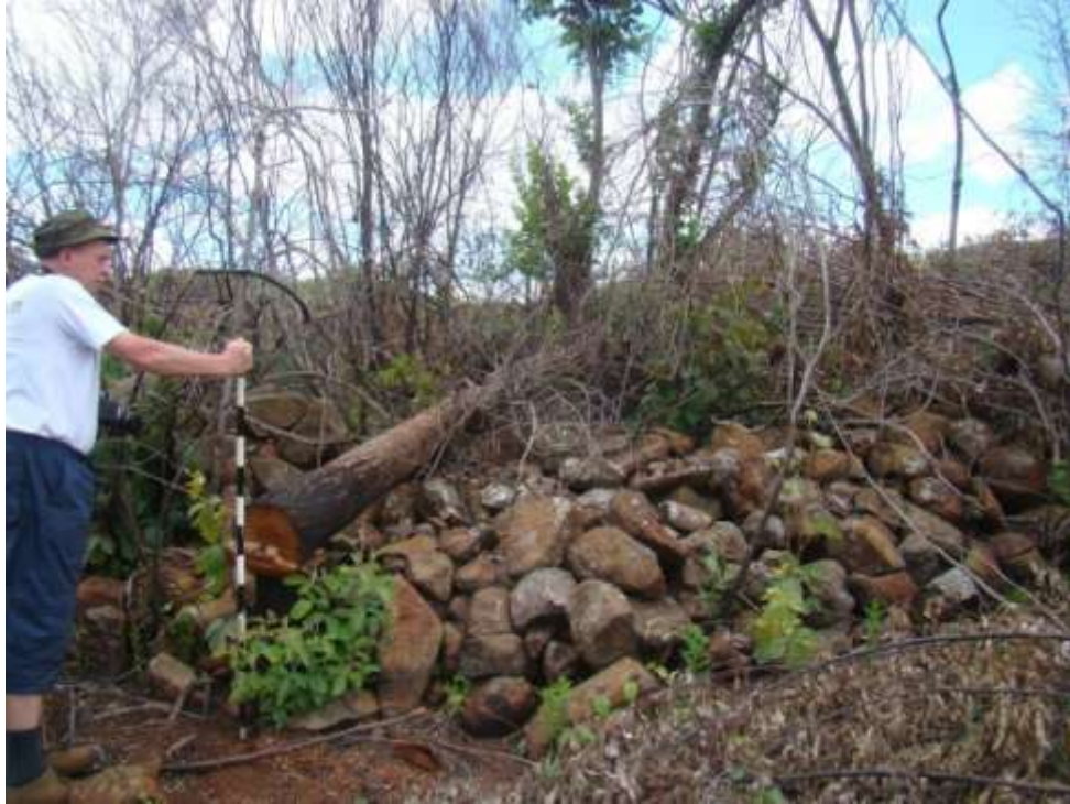
Fig. 250: C22 – 8: A circular wall on the northern side of the main access road is still in a very good condition, but damaged by a felled tree. The walls are in the region of 1000mm high.
