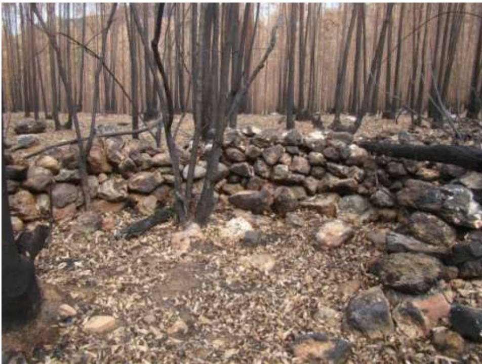
Fig. 186: Condition of a wall in this section.
