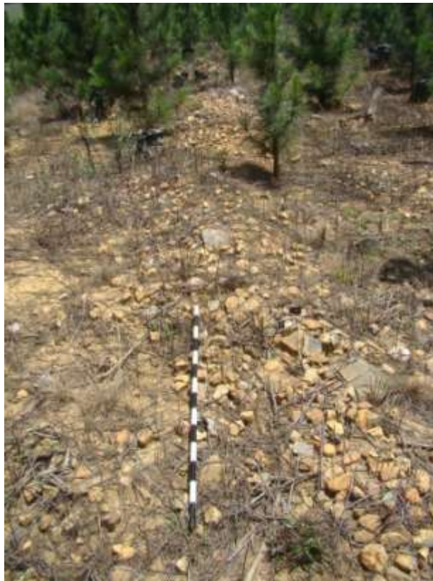
Fig. 14: The terrace wall which continues up the slope. It is deteriorated and located in a young plantation.
