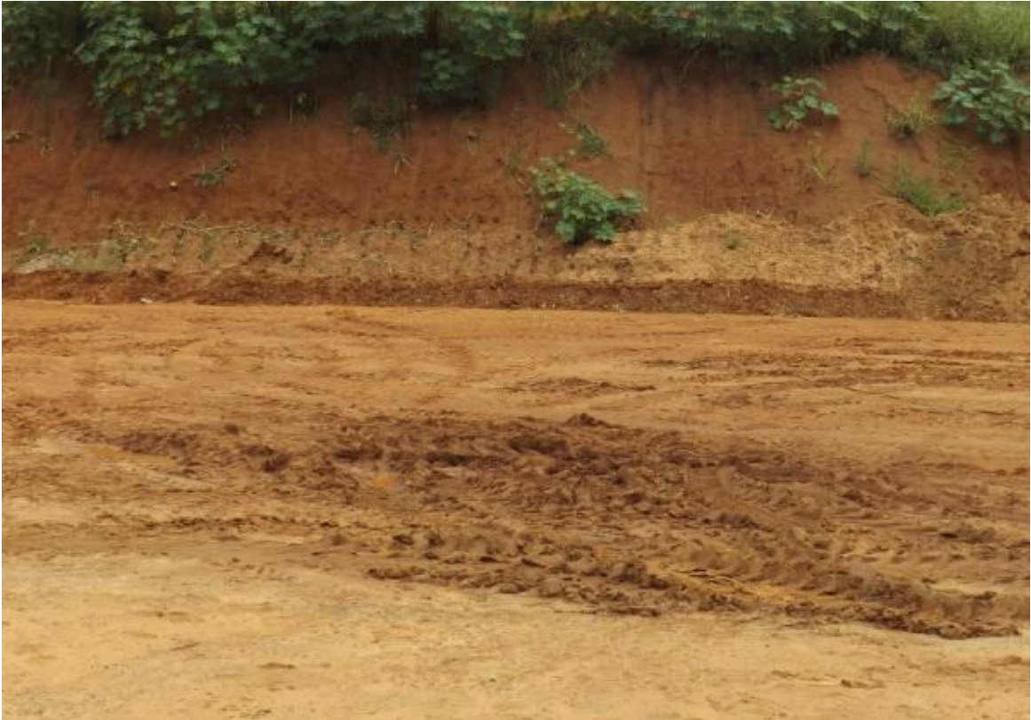
Figure 3: Earthcut from south of the development site, showing the characteristic appearance of the Umkwelane Formation (also known as Berea Red Sand).
