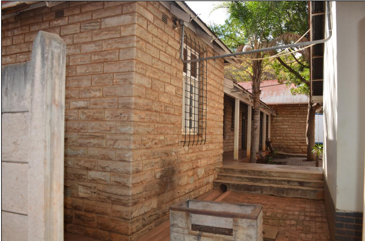
Figure 13. Disrepair at current building
