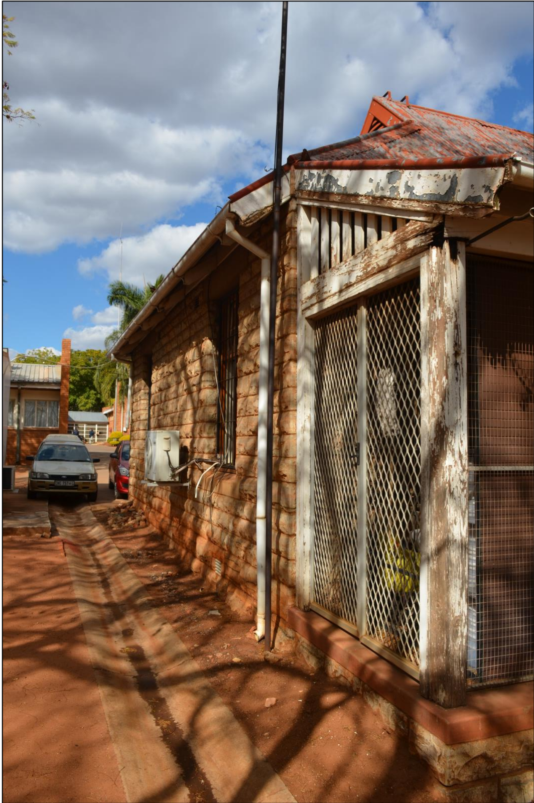
Figure 14. Disrepair in current building
