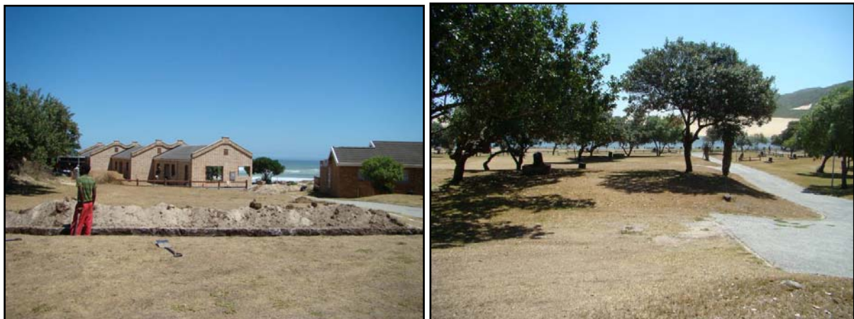
Left: The new chalets being constructed to the south-east of the estuary on the site of existing caravan and tent stands. Right: Kikuyu lawn covering the tent and caravan stands.
