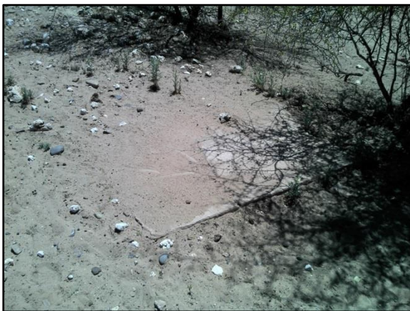
Figure 27. Dilapidated foundations of a structure
