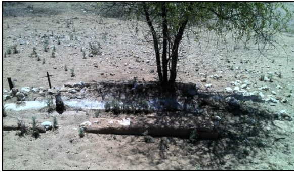
Figure 26. Dilapidated foundations of a structure
