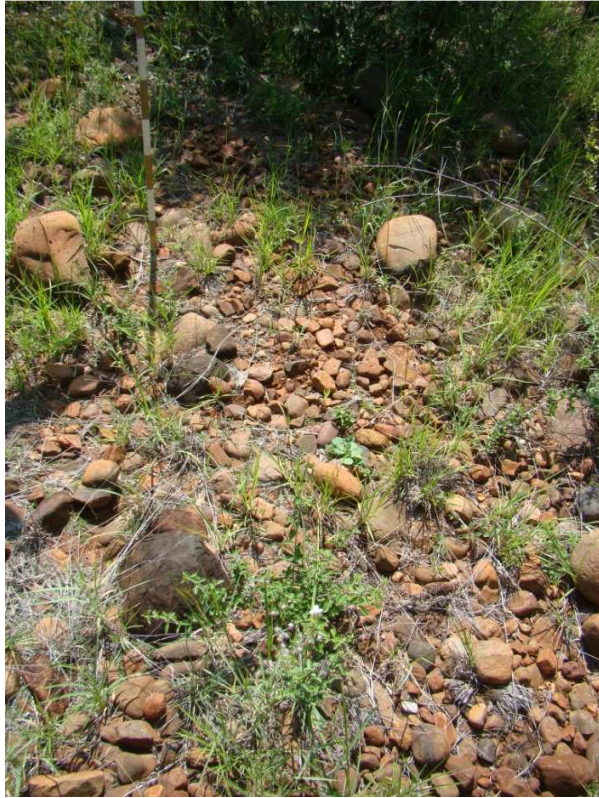
Fig. 15: Almost all the recent foundations are deteriorated or destroyed.
