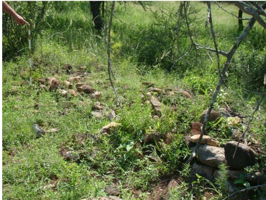
Fig. 11: A recent foundation is still visible but badly deteriorated.
