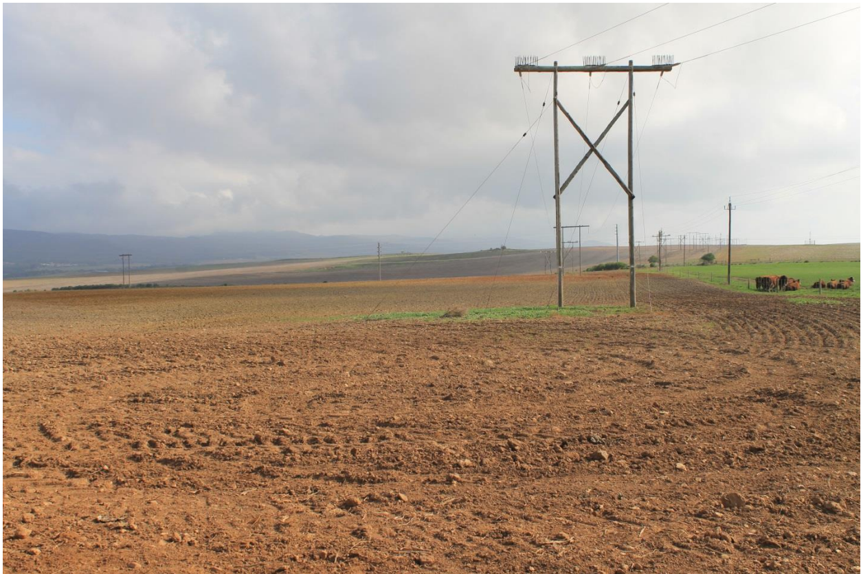
Figure 3 The existing 66 kV transmission line which is to be replaced with a new one. The landscape is typical of the area - gently inclined hills and cultivated lands.
