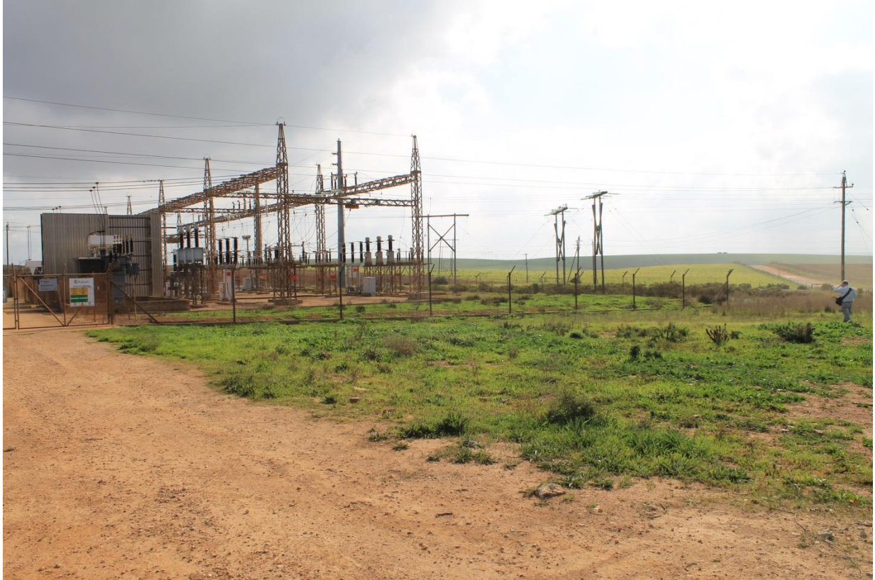
Figure 4 The existing Bredasdorp substation where the power line begins.
