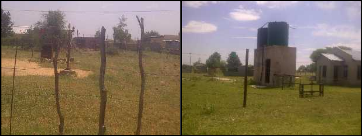
Figure 6- Old water supply infrastructure which include borehole and water reserve tanks
