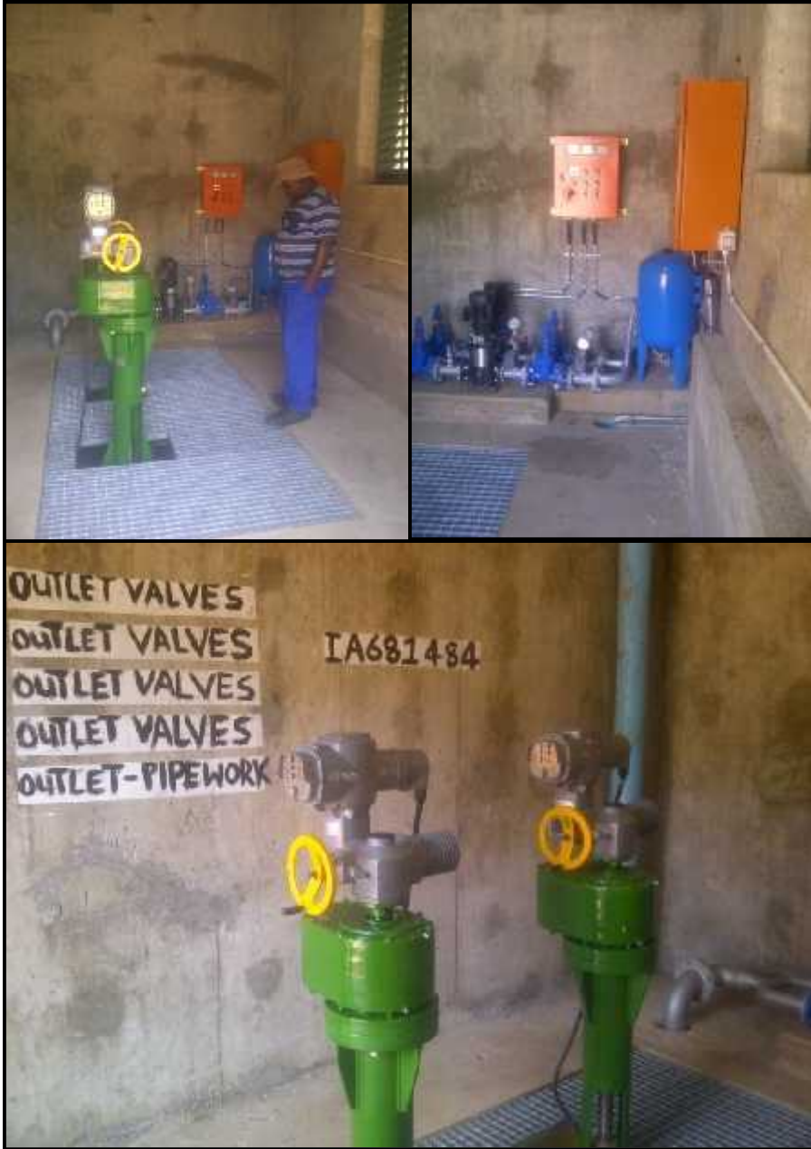
Figure 7- Existing water pump valves at Rust De Winter Dam
