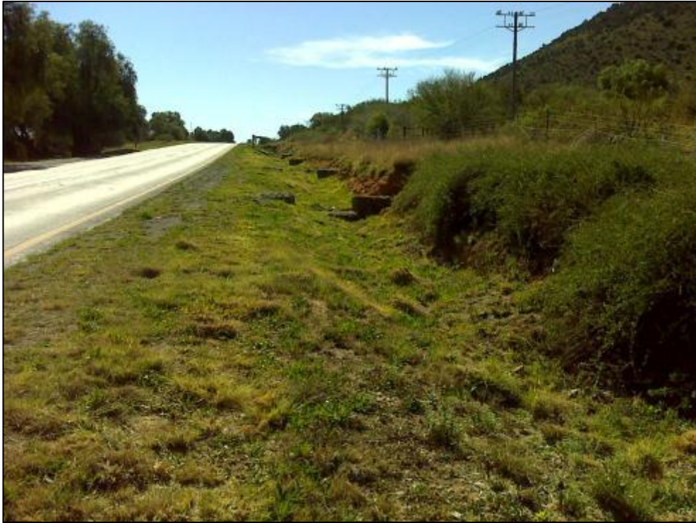
Figure 2-3: Various disturbances including water channels built within the road reserve and built-up, bulldozed sides.
