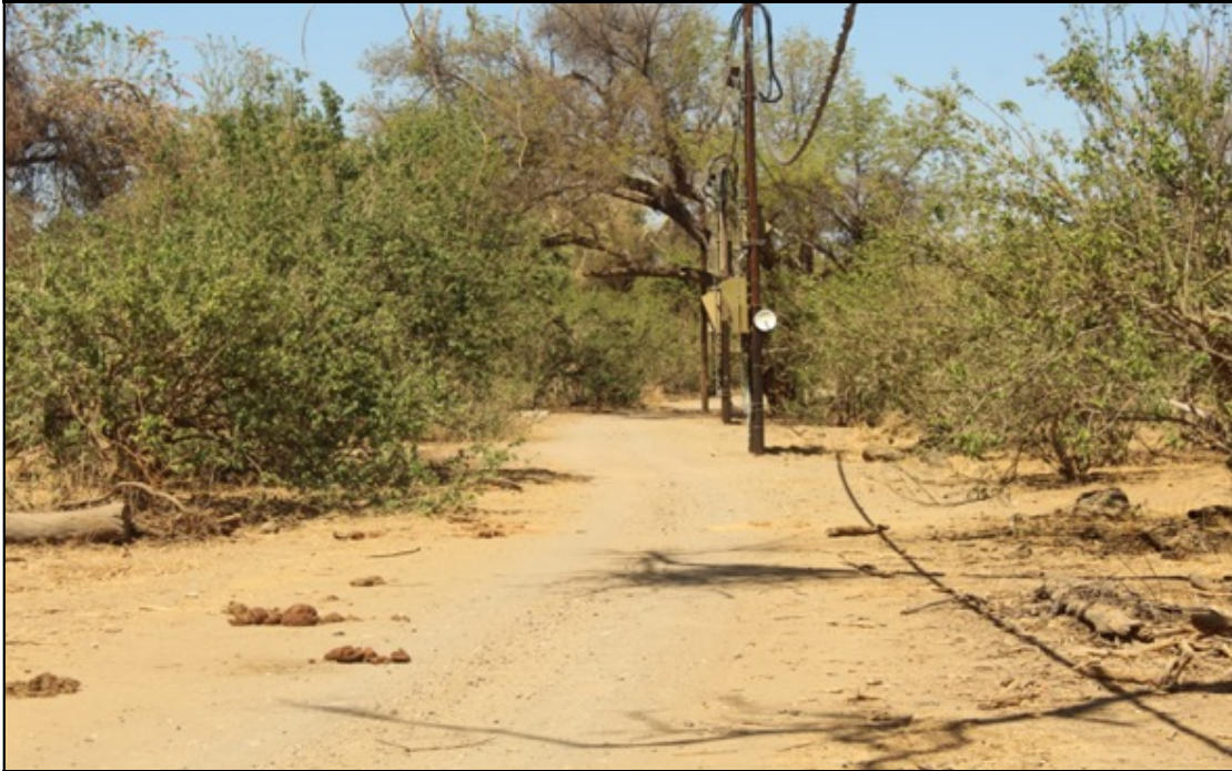
Figure 9: Electrical route alongside the gravel road
