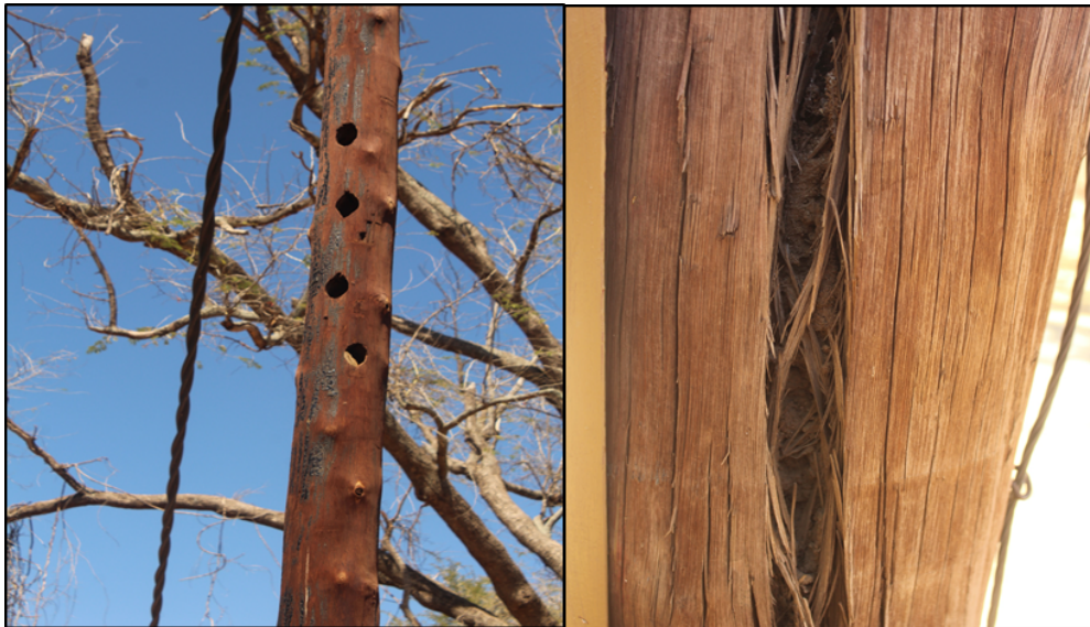
Figure 8: Wood parkers nest and termite's activities
