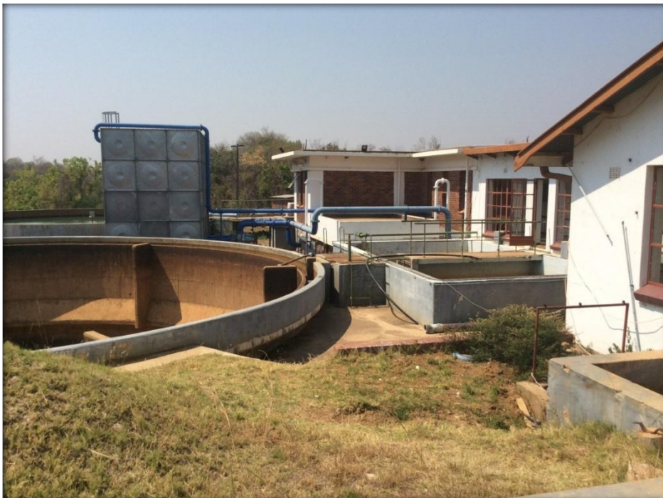
Figure 7- Part of the plant area showing the clarifier that is not in use and the filter beds
