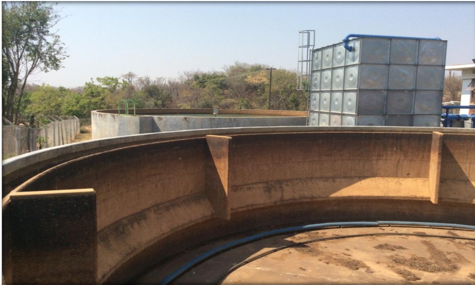
Figure 6-Two clarifiers at the WTW
