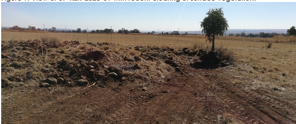
Figure 10: UP-KZK-2528-01 showing earth moving damage.
