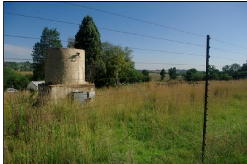
Plate 12: View of the Site CNRA-S1 tank with the dam in the background
