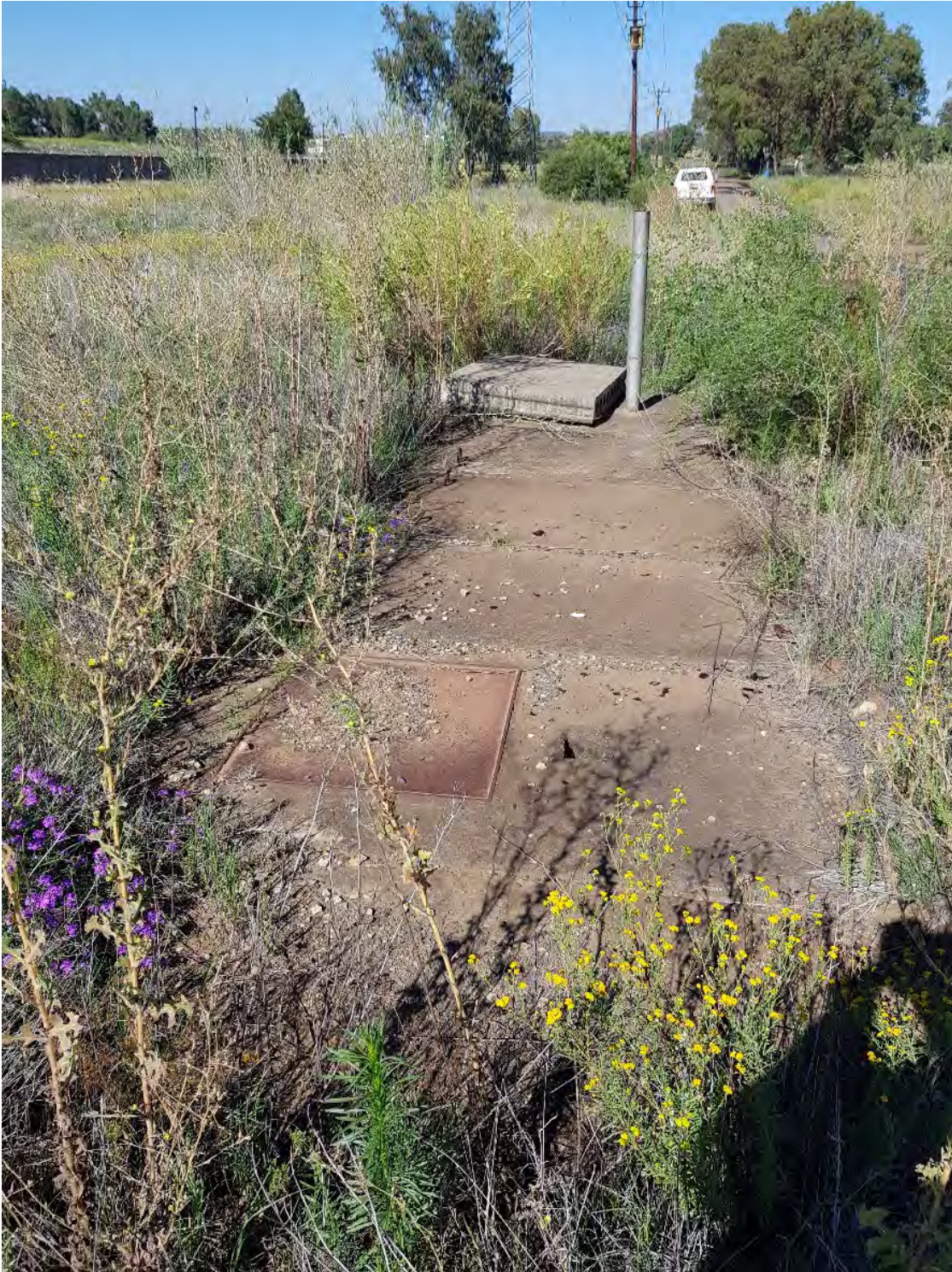
Figure 7: A second cement slab feature with metal trapdoor and breathing pipe S29° 04' 50.2" E26° 10' 56.5"
