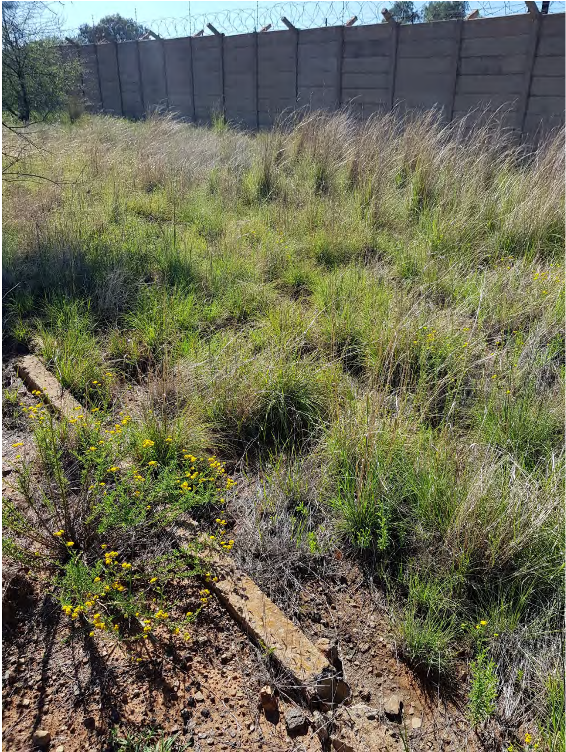
Figure 11: In situ section of the concrete structure which is presumed to have been a wall
