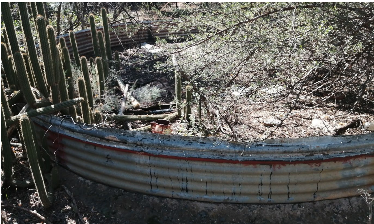
Figure 14: Corrugated iron walling of the dam rests on a course aggregate cement mix base
