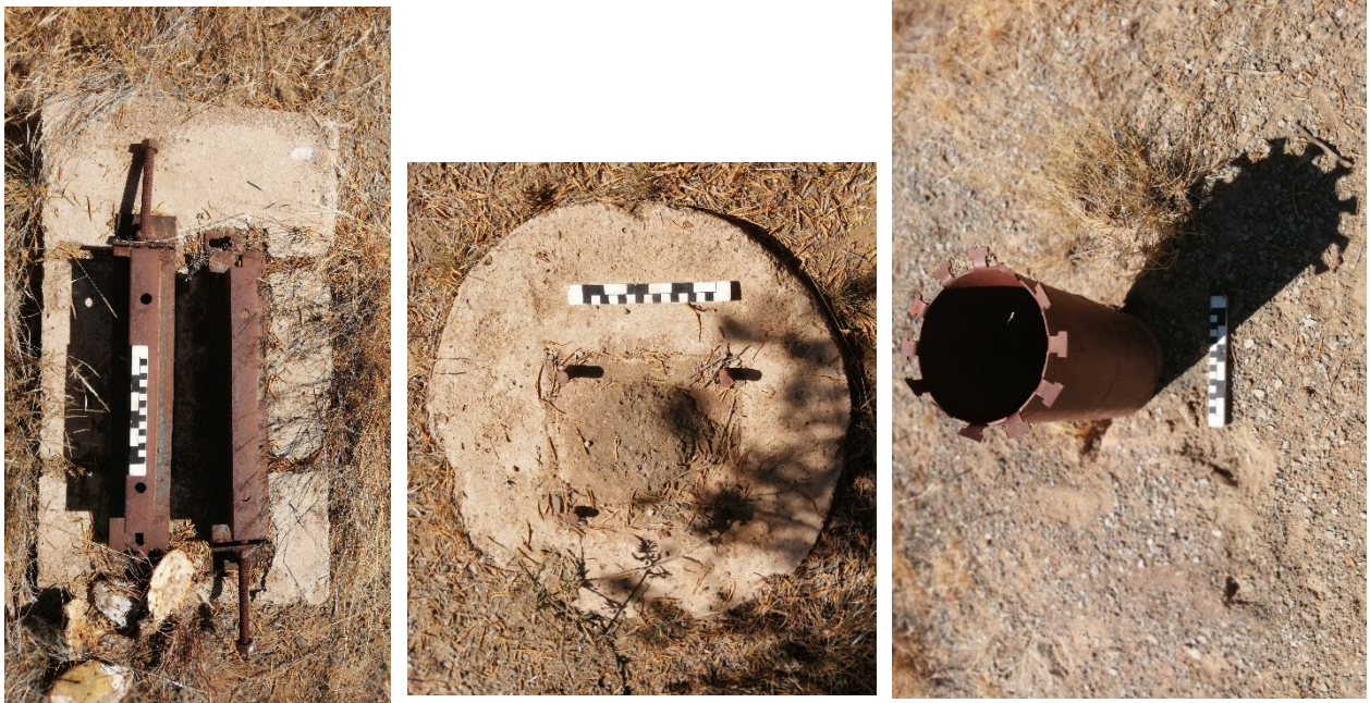
Figure 13: Indications of a borehole
