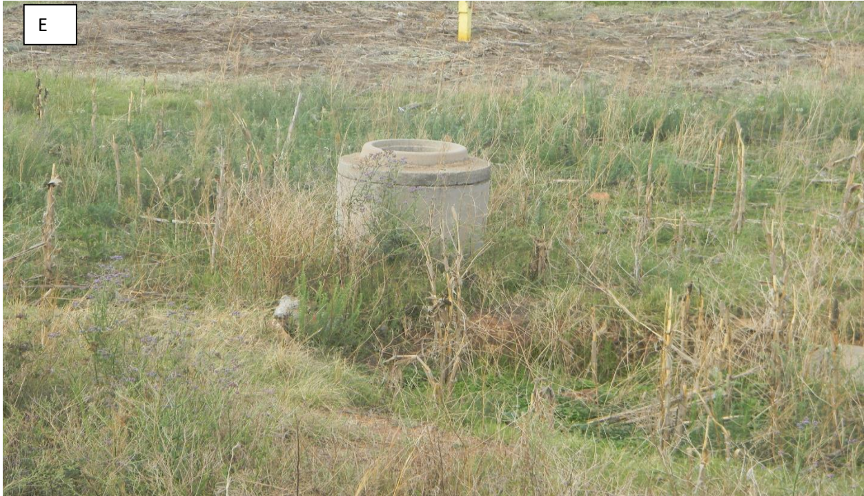
Plate 5: Photo E. showing bulk sewer pipeline infrastructure earmarked for upgrading (Author 2018).
