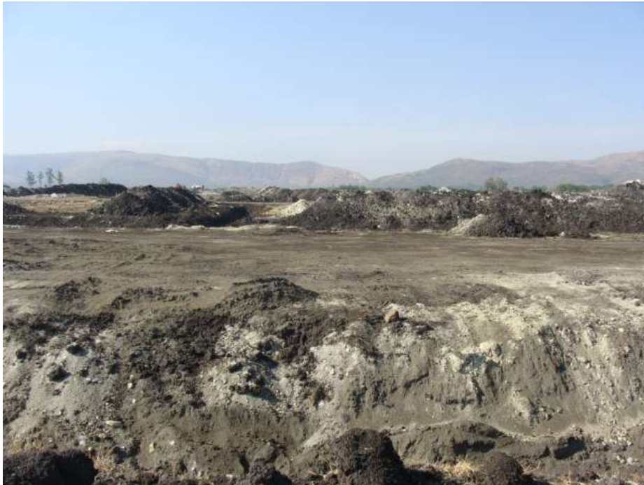
Figure 6: Southern section of the sewage line starts at this disturbed area.
