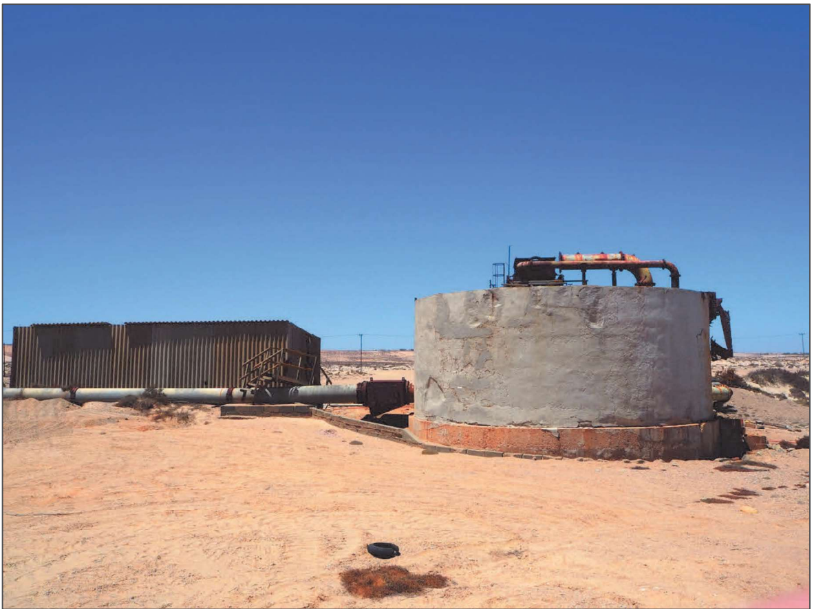
Figure 47. Pump Station and Reservoir
