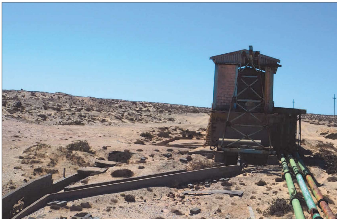
Figure 14. Second phase pump house
