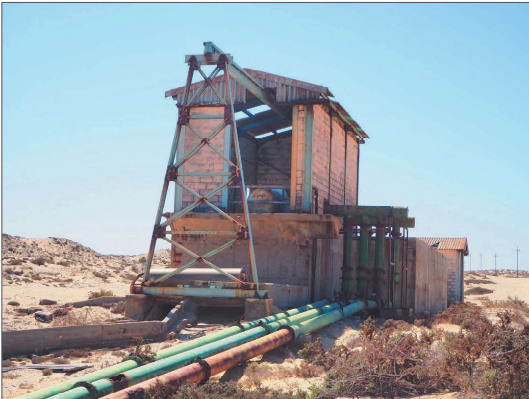
Figure 11. First phase pump station with gantry
