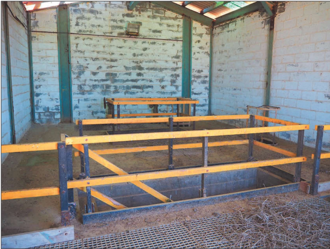
Figure 13. Inside of first phase pump house
