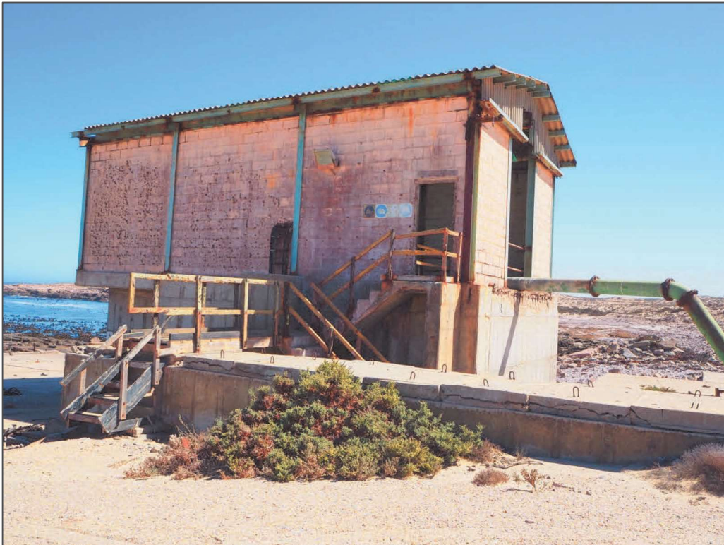
Figure 10. First phase pump station
