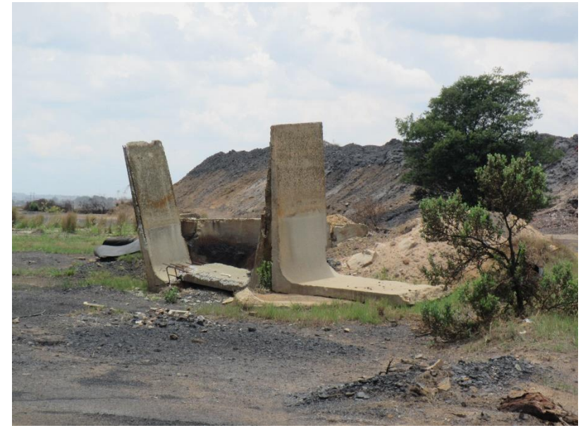
Figure 30 – View of more demolished remains
