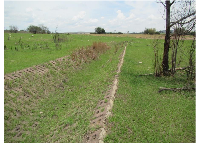
Figure 28 – Closer view of the ditch
