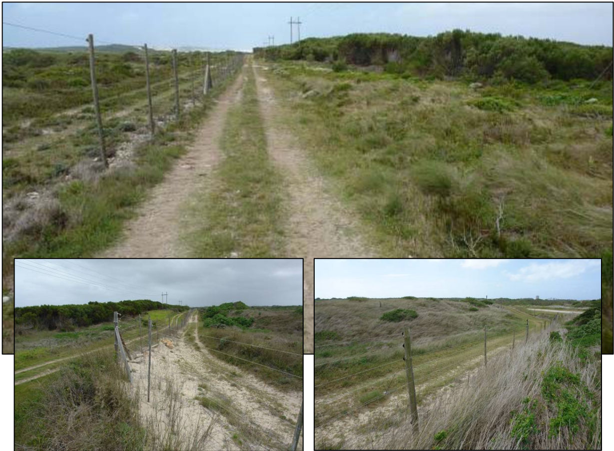
Figure 4. General views of the sludge pumping main route where it crosses Marine Drive and follows the boundary fence of the Nelson Mandela Metropolitan University's property in a westerly direction.
