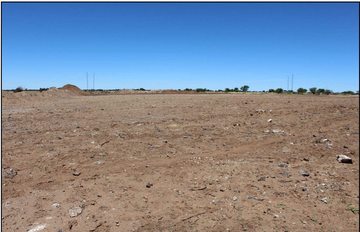
Figure 3: Clearings of the top soil in preparation to mine dolomite rocks, recent past activities
