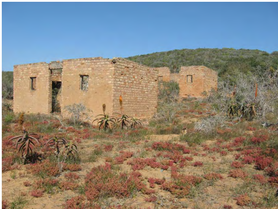
Fig.15 Two labourers' cottages, red clay brick, no roofs, no floors no windows possibly circa 1960 (Photos: J S Bennie)
