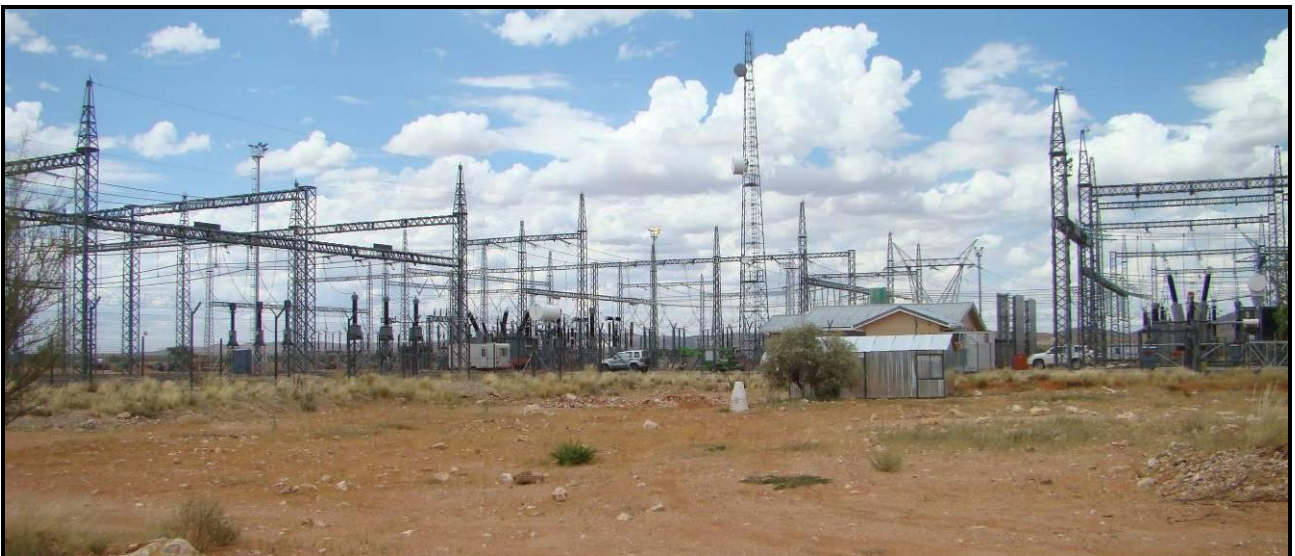
Plate 4: View of the Garona sub-station.
