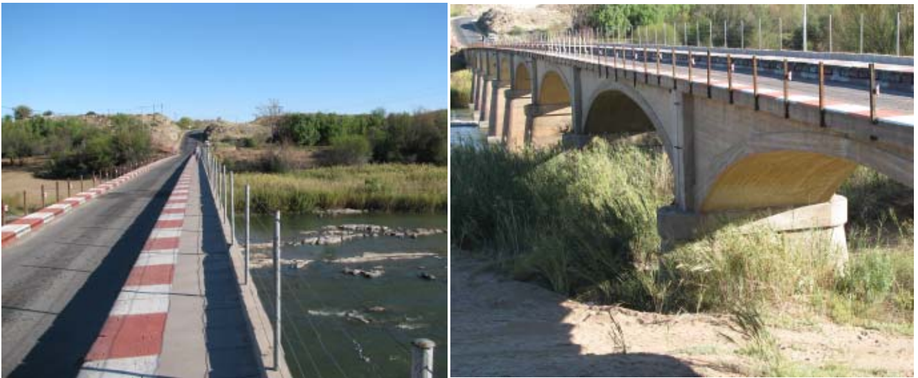
Plates 4 (left) and 5 (right). Views of bridge 2463 showing the pedestrian walkway and arches
