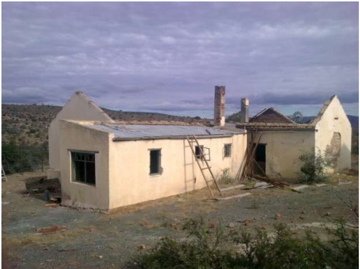
• Photo 10 Dilapidated Structure
