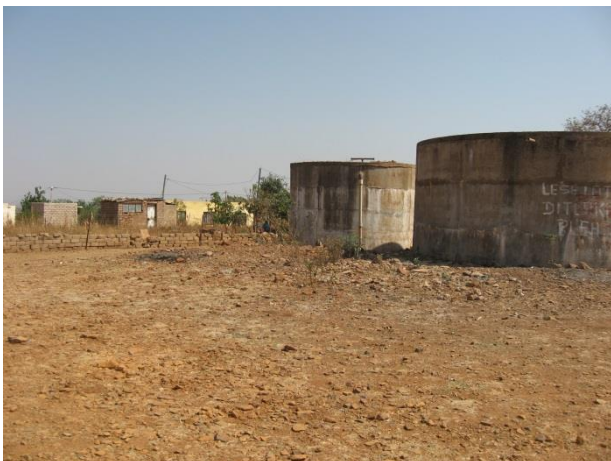
Figure 14 - View of the existing reservoirs and the location of Tshamahansi Reservoir B.
