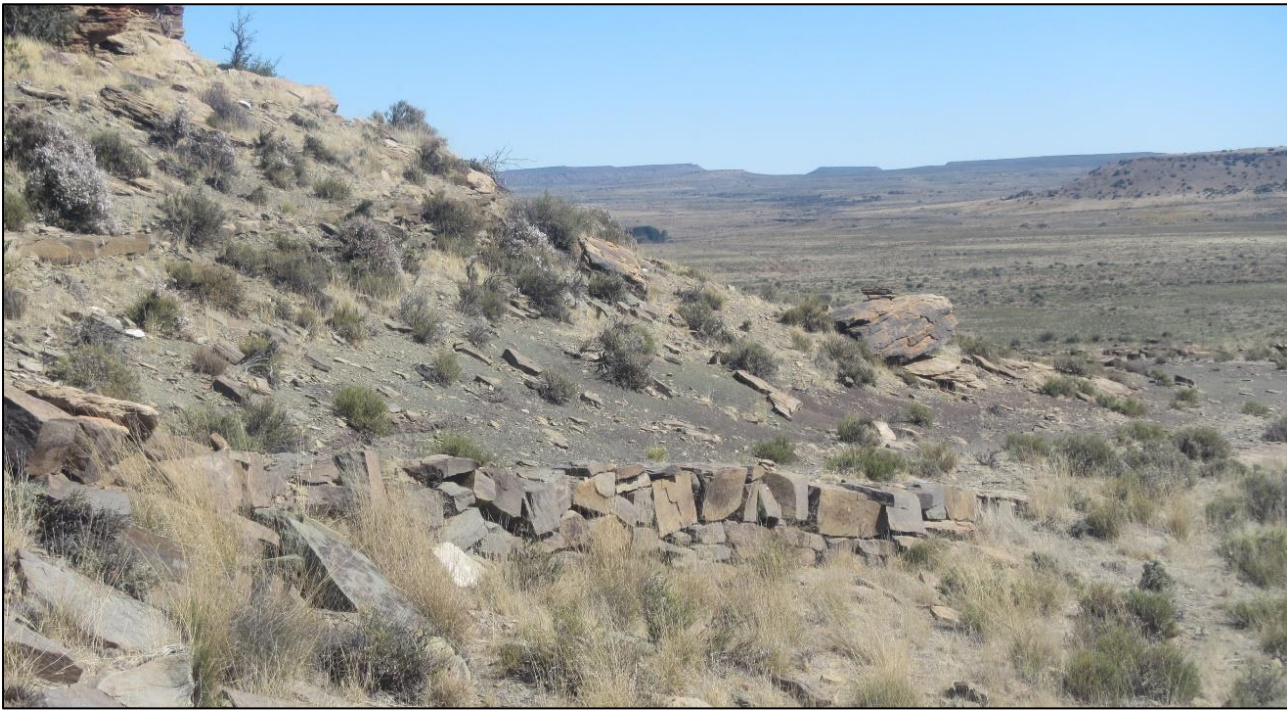
Figure 35: View of the stone retaining wall holding up the farm track at waypoint 213.
