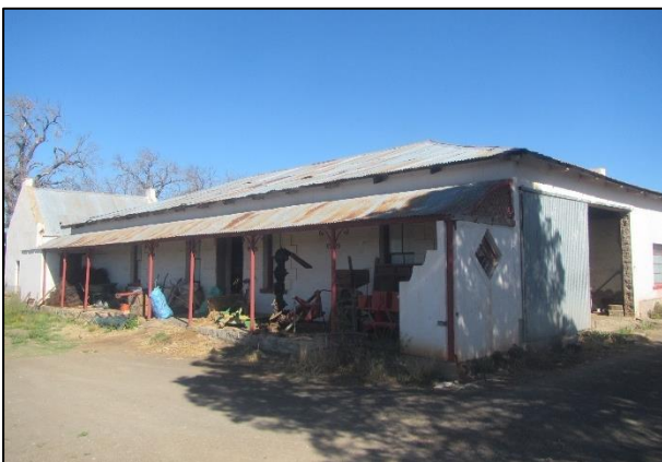
Figure 27: The southeast-facing front of the old farmhouse at waypoint 204. The north-eastern wall has had a large sliding door inserted. The gable in the background is a separate structure.
