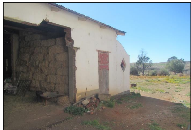
Figure 28: The south-western side of the old farmhouse at waypoint 204. A section of wall has been removed to facilitate large vehicle access.
