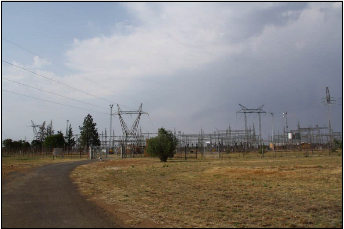
Fig. 5. The Watershed substation.
