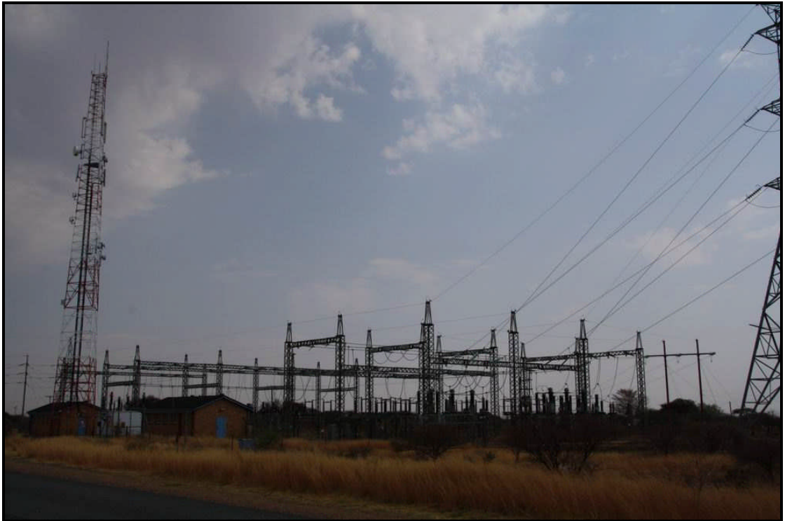
Fig. 3. The Mmabatho substation.
