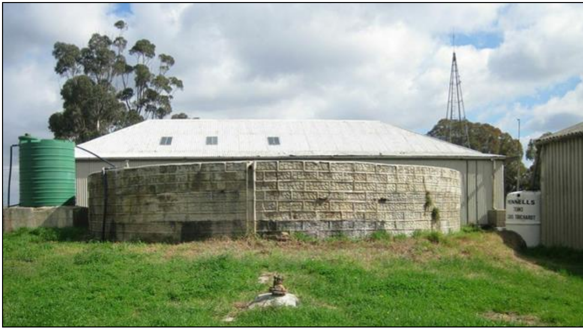
Figure 21: View towards the west of the decorative breeze block dam that predates 1951.
