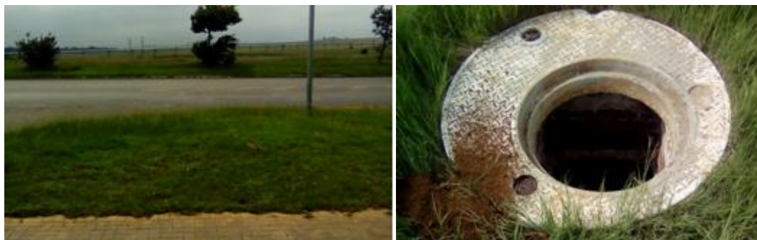
Figs. 13 and 14. Left. The view from marker 8 to marker 3. Right. At marker 3 there are two manholes. This is the first one. (Photo's S.M. Miller, February 2019.)
