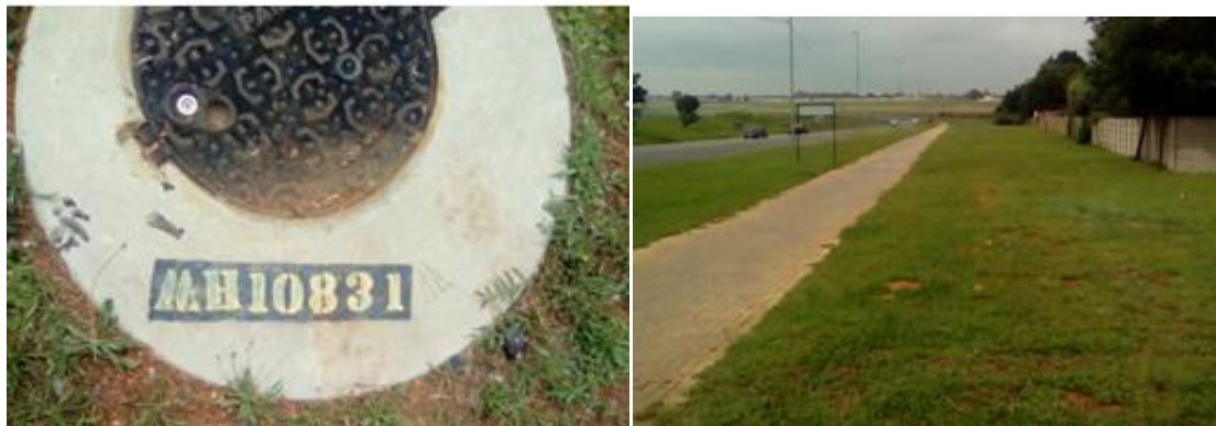
Figs. 11 and 12. Left. The existing manhole at marker 4 numbered MH10831. Right The view from marker 4 to marker 2. (Photo's S.M. Miller, February 2019.)
