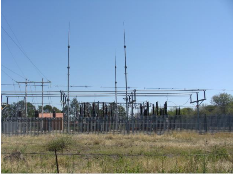
Figure 7 The Geluk Rural Substation.
