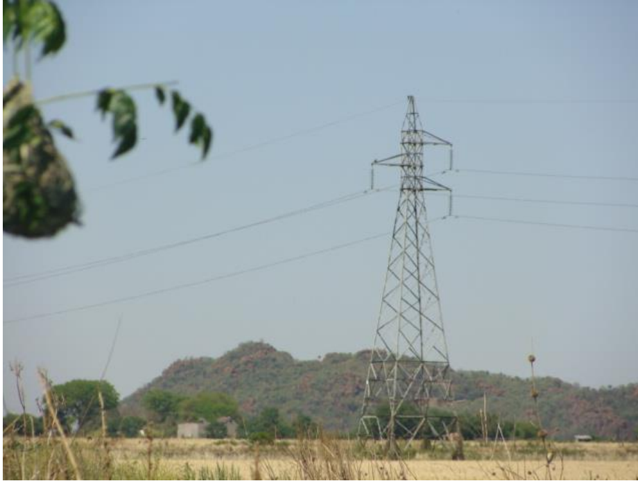
Figure 9 The power line along agricultural fields with which the proposed power line will link up.
