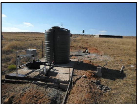
Figure 7.5. Water pump and tank.
