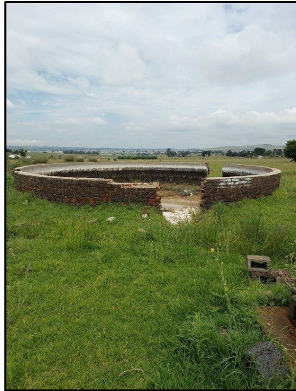
Figure 8-19. Existing degraded water reservoir situated near the foundations at EF004.
