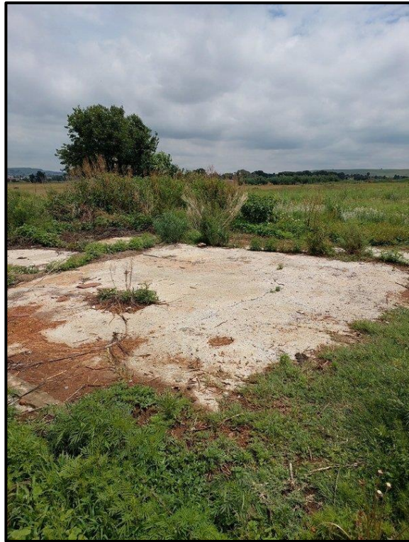
Figure 8-31. Small foundation situated on the western edge of the main structure at EF009.
