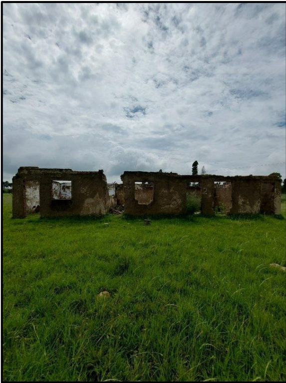
Figure 8-2. West facing wall of the degrading structure at EF001.
