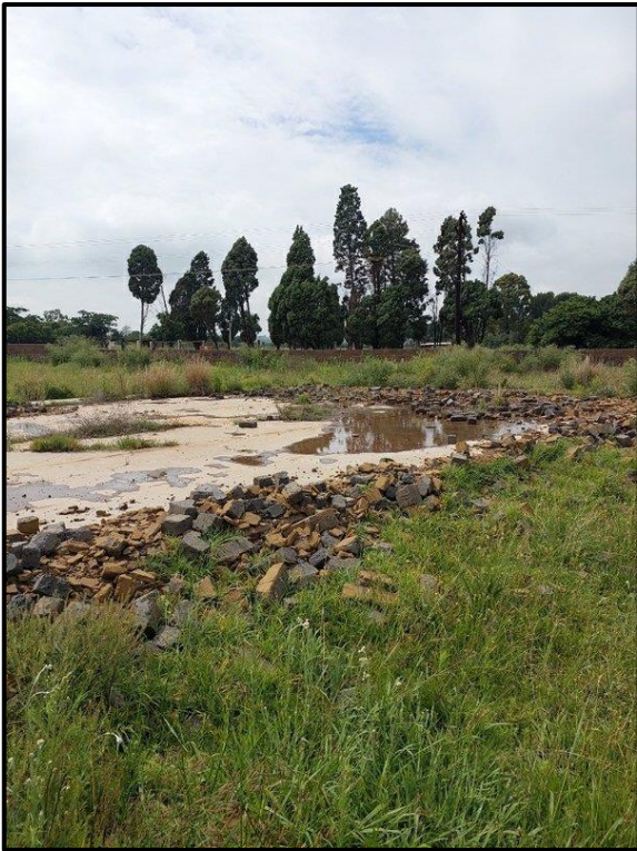
Figure 8-10. Large partially demolished foundations situated within the walled off area at EF002.
