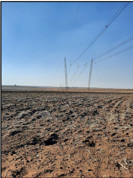
Figure 7.3. Existing powerline in cultivated area.
