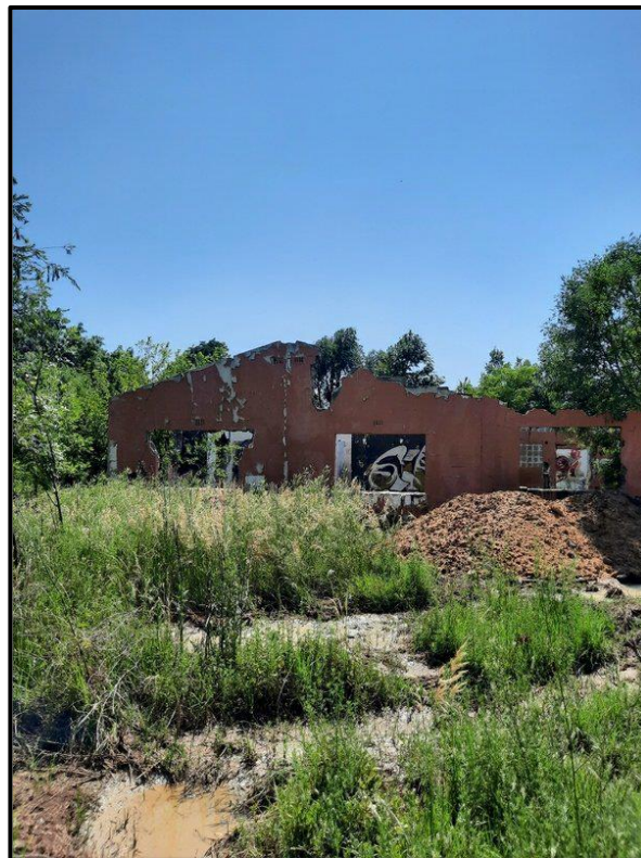
Figure 8.5. Waterlogged area around structure at Waypoint 235.
