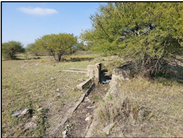
Figure 7.11. View of the degraded water canal along the western boundary of the Project area.
