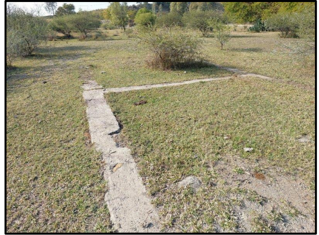
Figure 8.3. Broken down foundation at K001.
