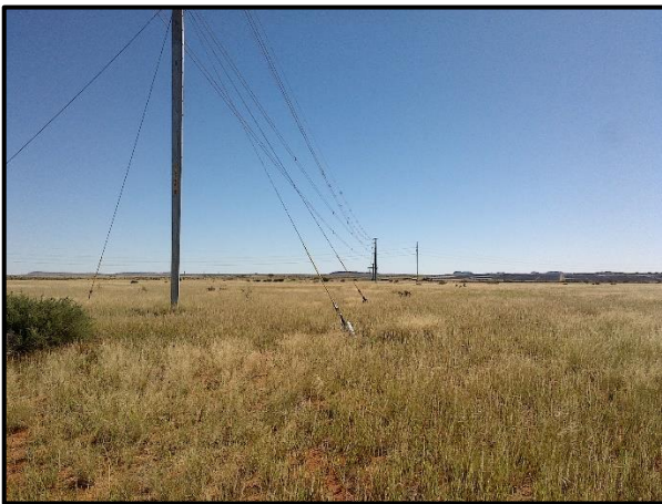
Figure 7.3. General site conditions and existing electrical infrastructure.
