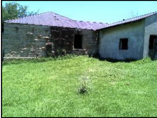
Figure 19. Structure with added on plastered sections.
