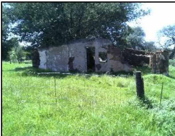
Figure 28. Dilapidated structure at KP 15.
