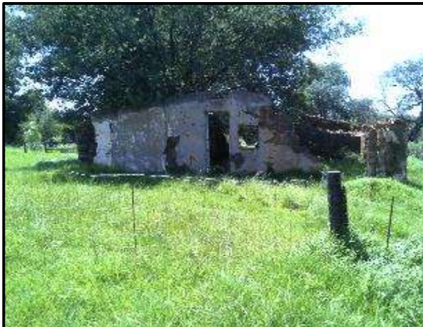
Figure 28. Dilapidated structure at KP 15.
