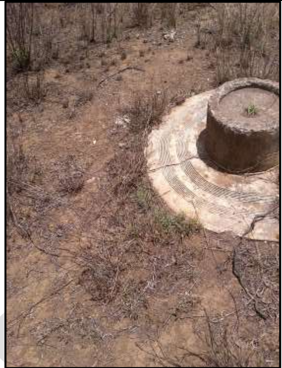
Figure 8-2. Existing infrastructure relating to water pipelines (possibly reticulation lines) noted in the study area.
