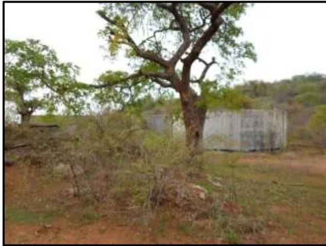
Figure 23. Existing water reservoirs
