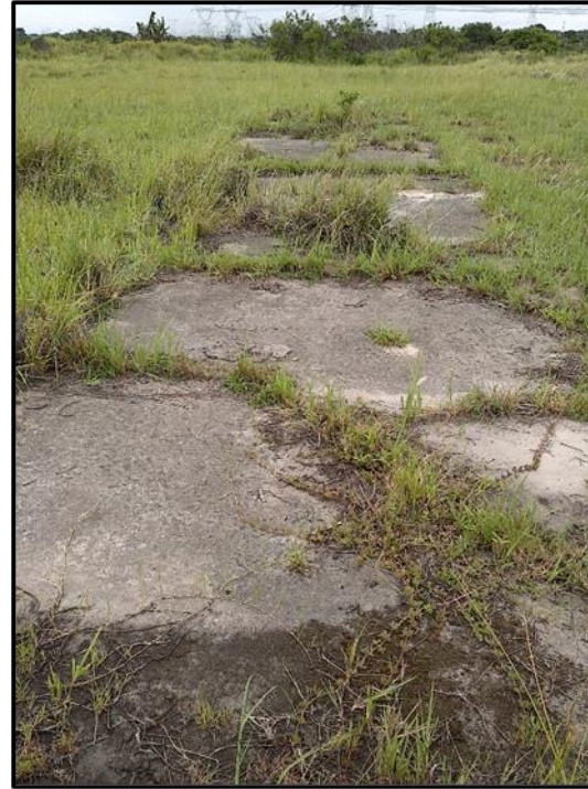
Figure 8-5. Figure 8-6: Cement slabs.
