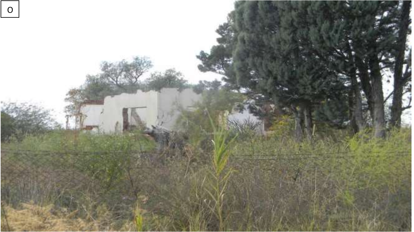
Plate 15: Photo O. showing demolished and dilapidated residential unit within the development site. Note that the age of the structure could not be determined during the survey.
