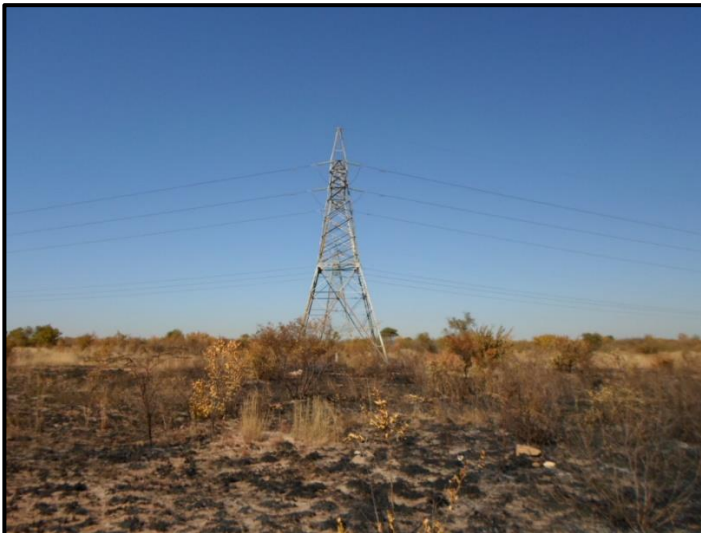
Figure 7. Power line on the South Eastern edge.
